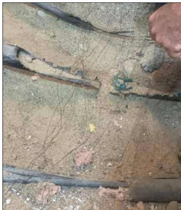
Burned electrical conduits that were under the slab.
