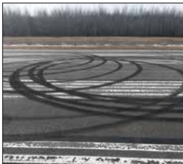
Recent damage to the Bigfork Municipal Airport runway.
