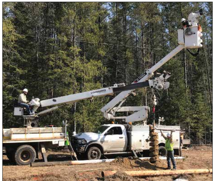
North Itasca Electric Co-op crews are rebuilding a 4.5-mile section of line along County Road 14. Here they are setting new poles and stringing new overhead line to accommodate the larger wire being installed.
